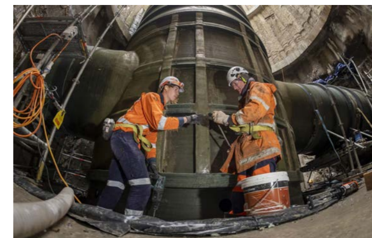
In-situ assembly and bonding of large fibre-reinforced polymer (FRP) pipe sections within an underground chamber on Auckland's Central Interceptor project.
