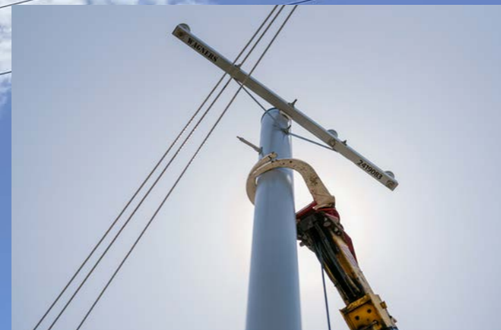
Wagners composite pole and crossarm assembly in service, requiring adapted installation methods and the use of elevated work platforms rather than traditional spike climbing.
