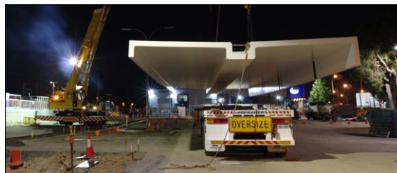
Kenwick Station composite roof 7Jun. A single piece sculptured monocoque canopy designed for durability and rapid overnight installation. Capital House Australasia Perth, made by Swarbrick Technologies. Image courtesy B Nelson
