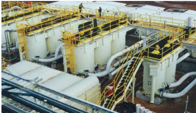
Spent Electrolyte Tank installed at Cause Nickel, Kalgoorlie
