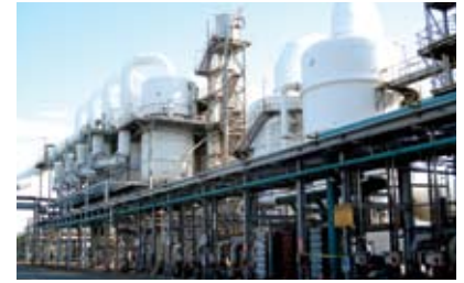
L-R 4 x 2 GRP Electrostatic Mist Preceptors 6.5 m diameter x 18 m high, halide tower and gas cooling tower
