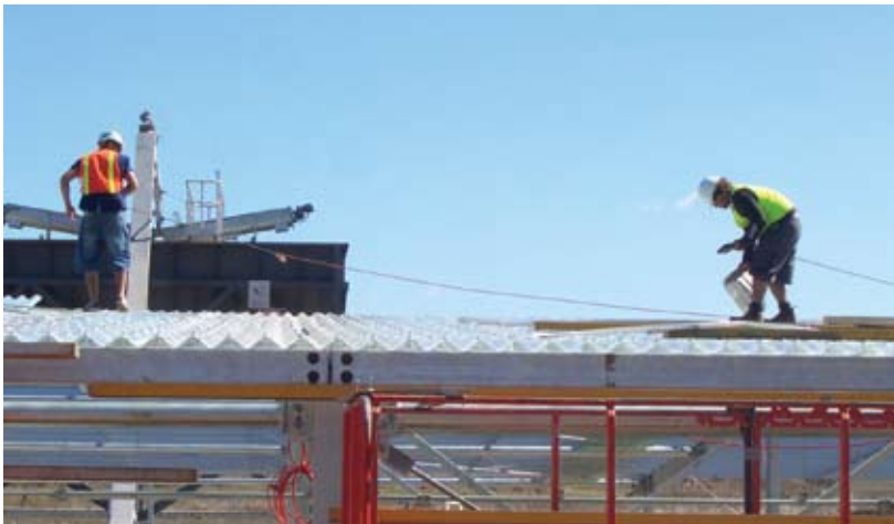
'Wonderglas GC' clear fibreglass roof sheeting installed at the Toowoomba Sludge Drying Facility
