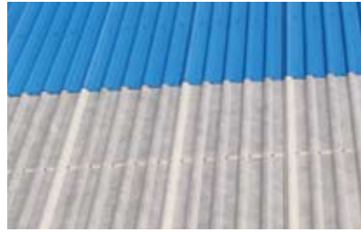
'Webglas GC+' fibreglass roof sheeting and wall cladding installed at Xstrata Townsville Copper Refinery
